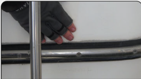
Photo 18: Exposed gelcoat area.
