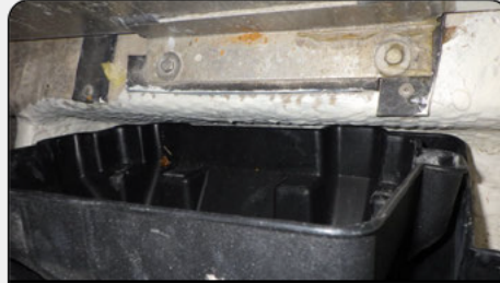
Photo 5: Battery cover not in place
