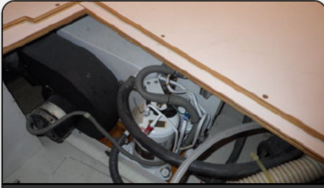
Photo 19: Rusty water building up in the HVAC drip tray
