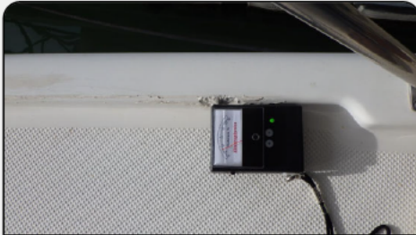
Photo 17: Poor quality repair but no water intrusion at this stage. Note slight crazing on toe rail on LHS of photograph
