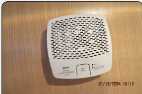
Photo 1: Xintex CO detector in aft cabin was not powered up and did not test
