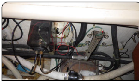
Photo 34: Steering hydraulics again but note good bonding wire to lever and general cleanliness
