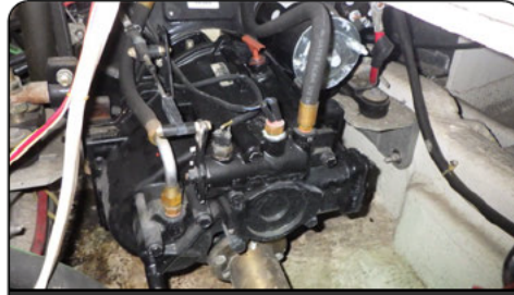
Photo 32: View of port engine from aft cabin. Note engine mounts in good condition and minimal corrosion
