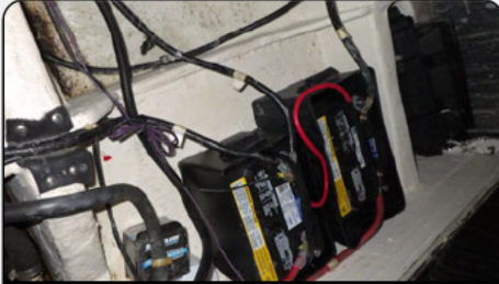
Photo 4: Port battery bank. No covers on terminals and on stbd battery a small black wire is sighted under large cable. No overcurrent protection within 7 inches.
